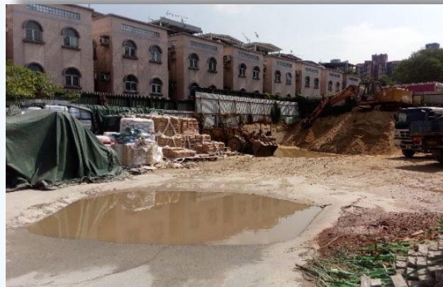
Piling up of Construction Materials in Open Storage near Residential Developments
