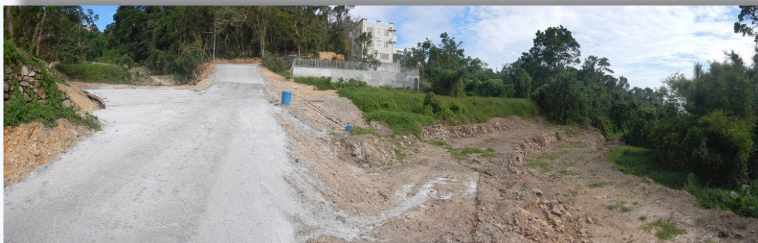
Unauthorised Excavation and Filling of Land in an Area Zoned 'Green Belt' in Clear Water Bay North, New Territories, before Enforcement Action
