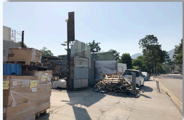
Unloaded Materials and Vehicles blocked the Pedestrian Paths and Entrance of a Brownfield Site
