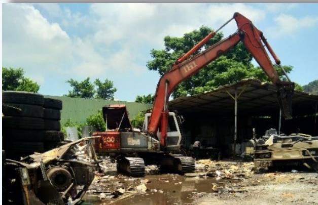
Brownfield Operation may cause adverse Environmental Impact and Visual Intrusion
